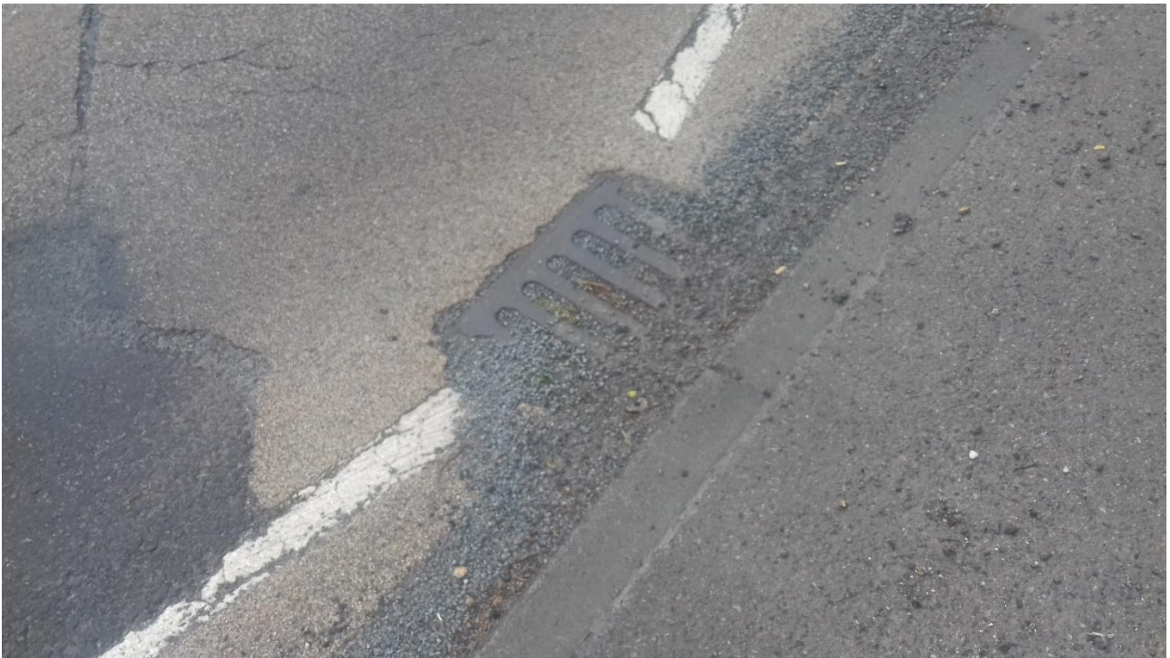
Highways Ref 359879 Blocked Drain by Traffic light crossing by TNRC
