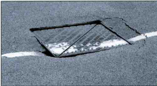
Unsafe water board man-hole cover on Thanington Road
