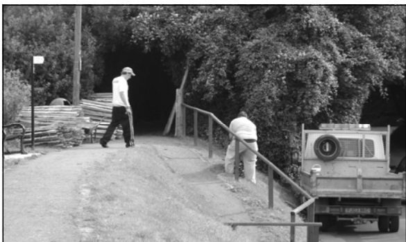
Contractors deliver the fencing. Top, first stage of the project is completed on time
